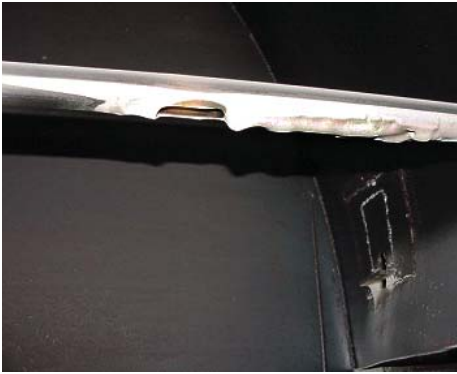
This photo shows the typical fly ash buildup on the downstream side of the K-Bar 2000B Sensor Support Tube.
